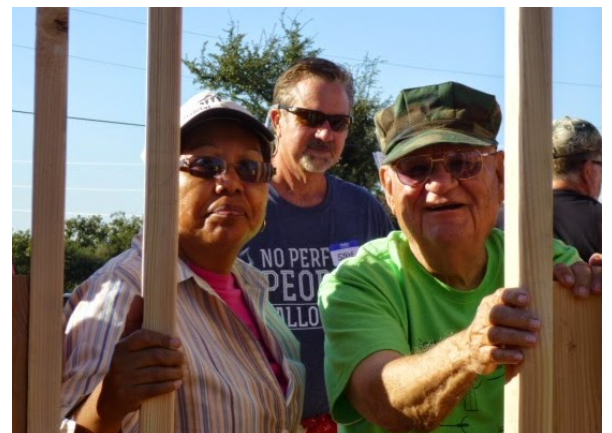
Roberto and Celina Canales raising the first wall of their new home.
